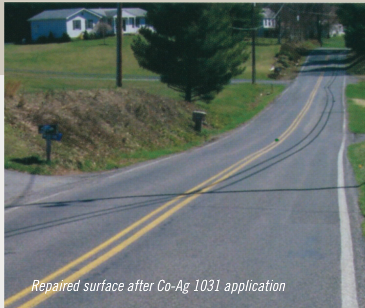
Excessive bleeding on road surface
